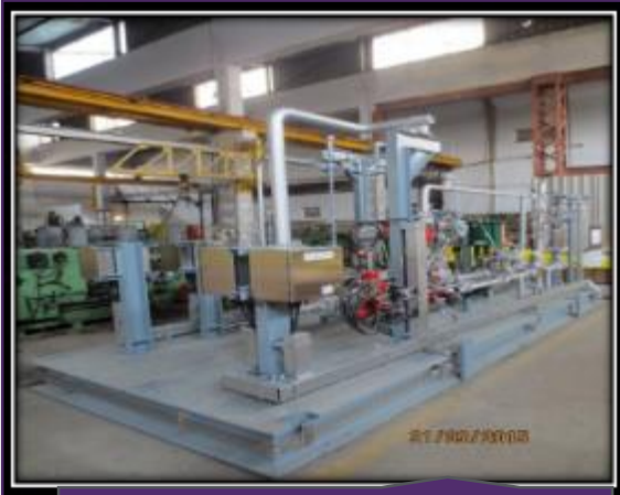
Fuel Gas Skid. NSRP, Vietnam
