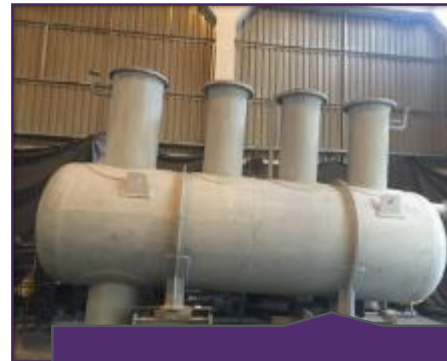
Glycol Drain Drum
