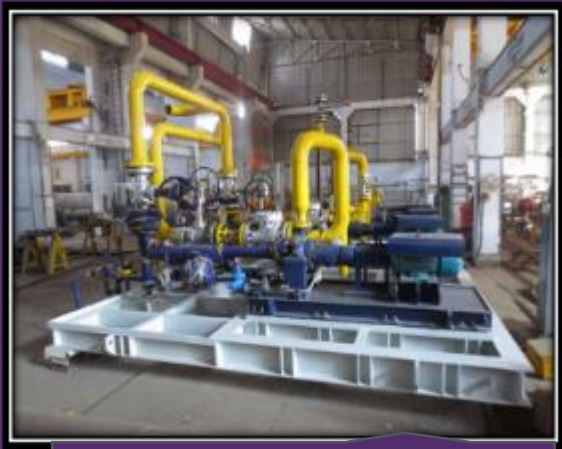
Pump Skid, IOCL, Paradip
